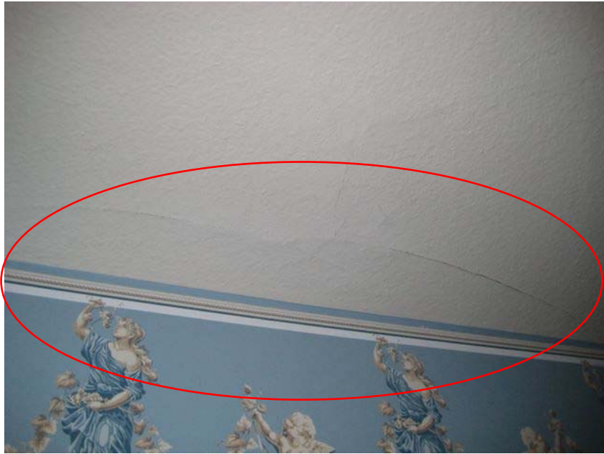
Picture Five – Bathroom water stain crack unfixed
