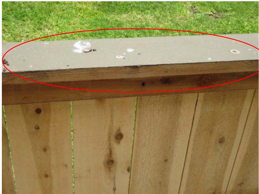
Picture Four – Unweathered Proofed Fence covered in bird droppings
