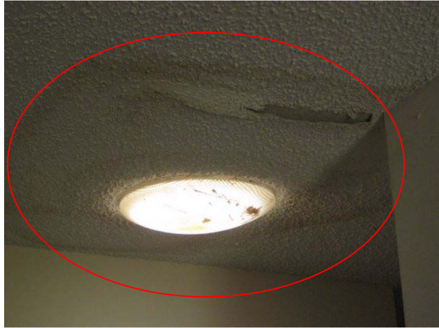
Picture Six – Picture Hall water stain with hanging stucco
