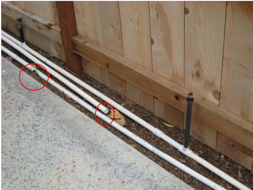
Picture Three – Broken Pipes
